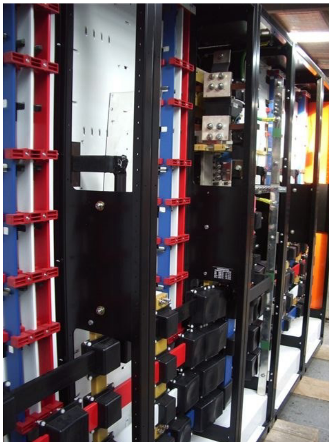
Typical rear sections of switchboards showing busbars insulated by rigid sleeving and busbar joint covers
